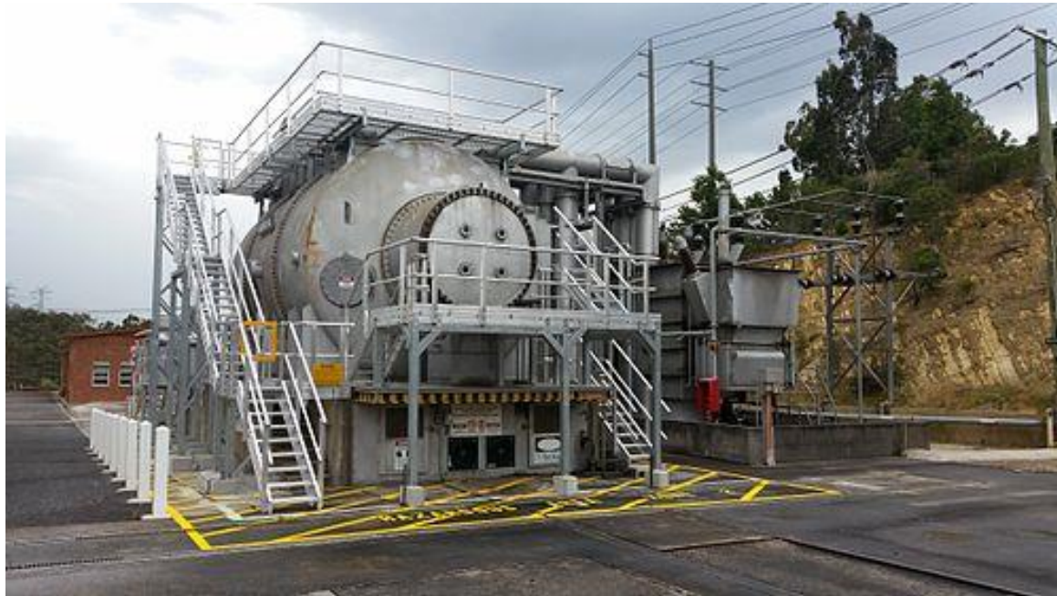
FIGURE A.4: Synchronous Condenser
